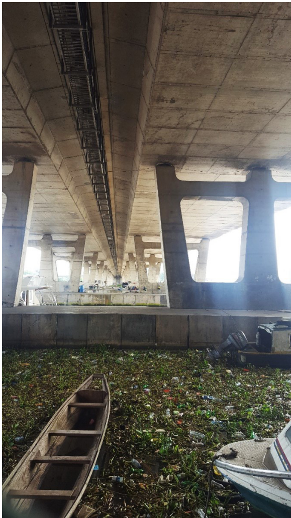
Beneath the bridge: The Third Mainland Bridge is 11.8km long and handles 7 000 vehicles a day – vital infrastructure. Still, it is often congested and poorly maintained
